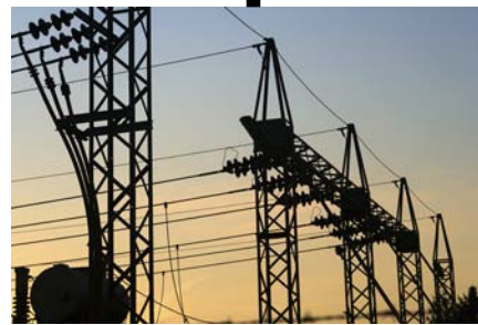
Utility Company AC Power
